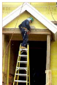
Improper use of the top rung of a ladder
